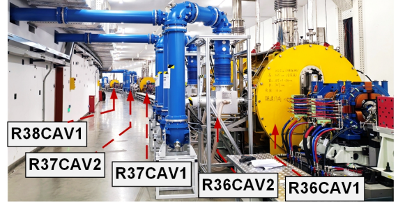
Figure 7: Five 166 MHz modules installed in the HEPS.
