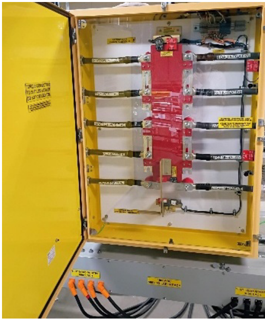
Figure 6: DPSS transfer switch
