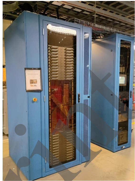
Figure 4: Auxiliary DPSS and control racks
