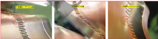
Figure 4: The discoloration was observed at the comb structure inside the D11 bellows.
