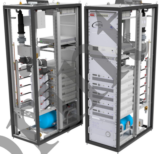
Figure 1: Solid State amplifier for the first buncher cavity, as built.
