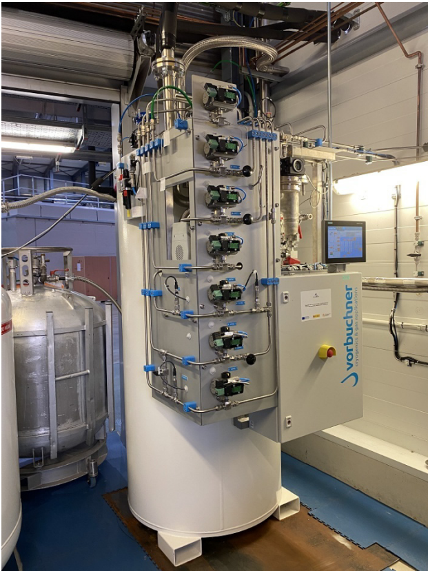
Figure 3: Purifier installed in the ALBA helium recovery plant.
