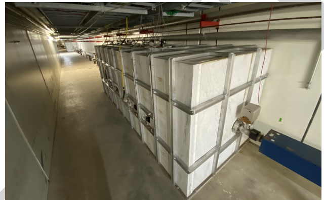
Figure 3: New MI8 collimator installed at station 827, the other installation is seen in the distance at location 825.
