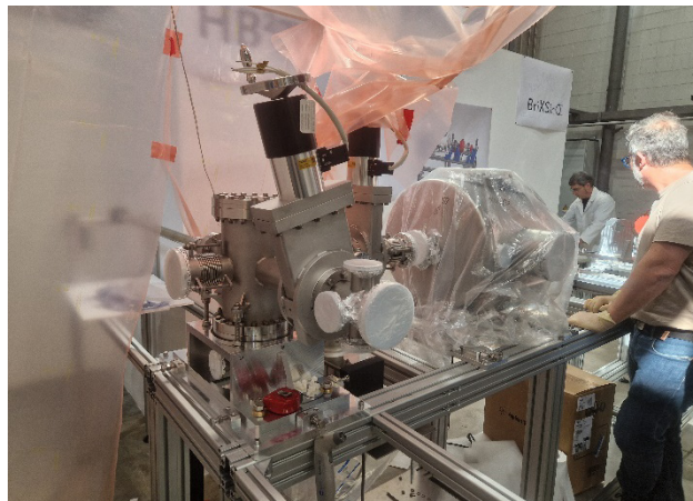
Figure 2: Status of the vacuum system and DC gun chamber installation in May 2026.
