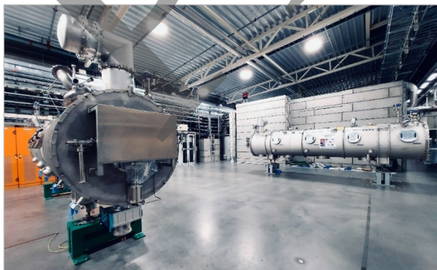
Figure 3: TS2 area with two slots available (Preparation 1 and Preparation 2). Elliptical cryomodules already in place.
