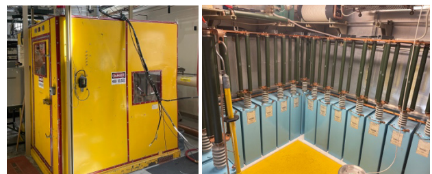
Figure 4: Outside photo of the capacitor bank used in the current amplifier test stand (left) and capacitor arrangement inside bank (right).
