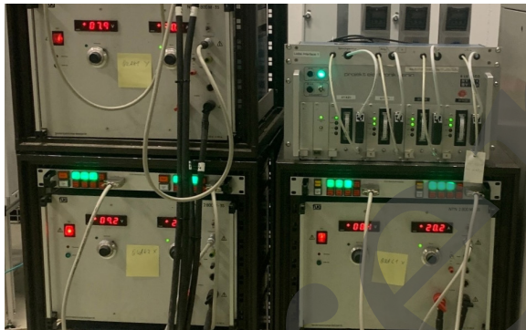
Figure 3: Refurbished FUG power supplies with new developed interlock interface to the Beckhoff-PLC.
