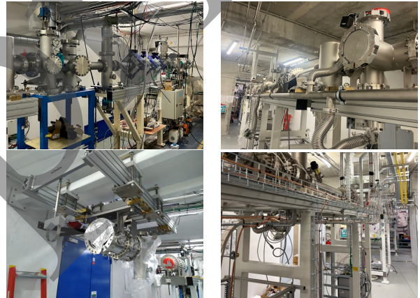
Figure 5: Photos of the current assembly in the "salle aux piliers" for the LT section 2.
