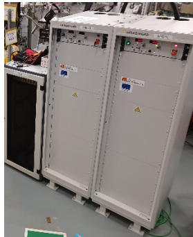
Figure 5: High voltage power supplies.
