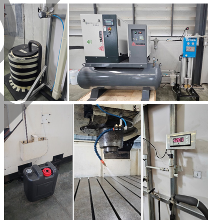
Figure 3: Ethanol spray cooling system installed at N.K.R. Engineering Company for oil-free five-axis CNC machining of the VCB-4 chamber halves.
