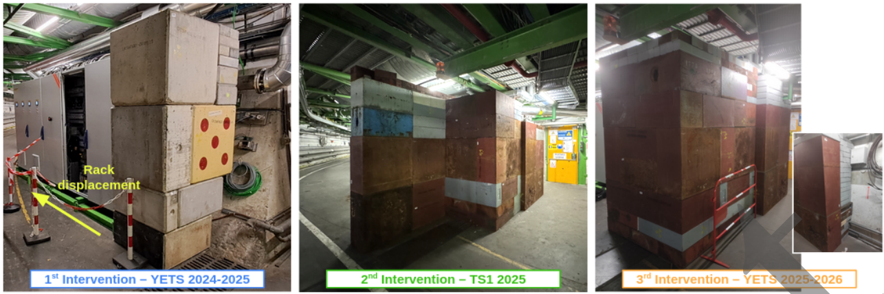
Figure 1: Evolution of the shielding configuration implemented by three interventions to protect the AMB system rack from radiation streaming at the UL84 entrance.
