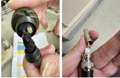
Figure 8: Examples of sensor and connection issues, including a degraded connector and a damaged BNC adaptor.
