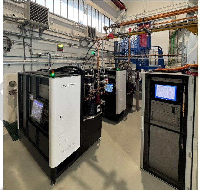
Figure 2: The 25MW X-band source and the 22MW C-band source installed in the final position.
