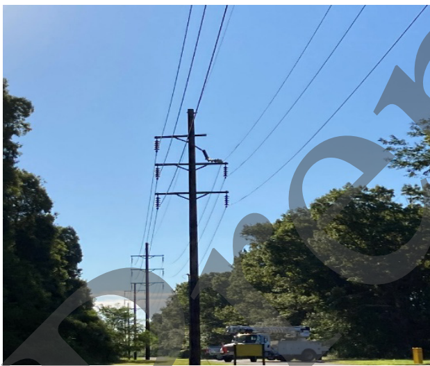
Figure 3: Power line arm failure for the main AC feed to RHIC.
