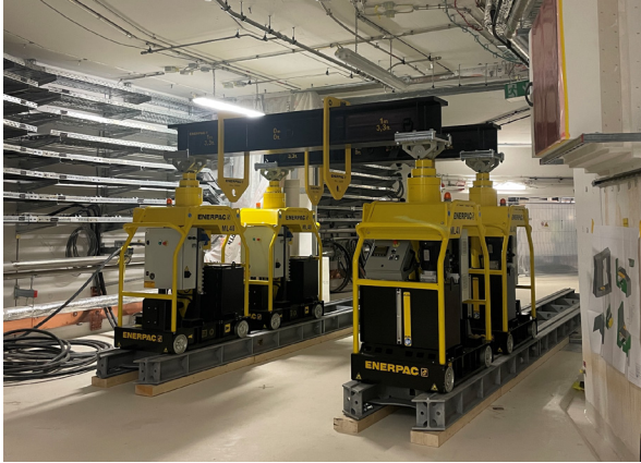
Figure 6: Hydraulic transport system for lifting the beam-line components over the building joint.
