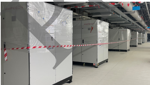
Figure 11: Power supplies of the RF acceleration system in SIS100.
