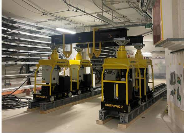
Figure 6: Hydraulic transport system for lifting the beam-line components over the building joint.
