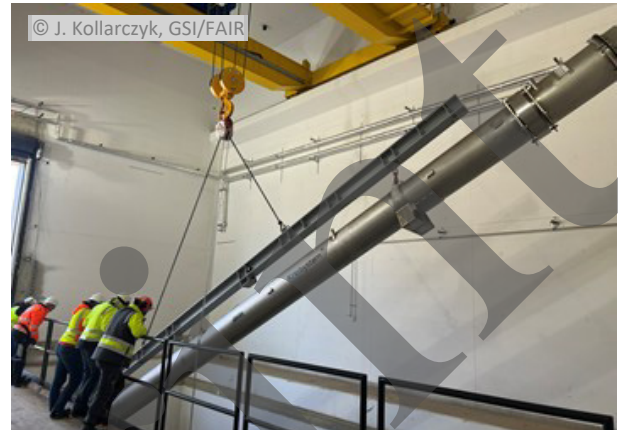
Figure 12: Lifting of a 13 m long section of the cryogenic bypass line connecting the cryogenic components across the warm sections.
