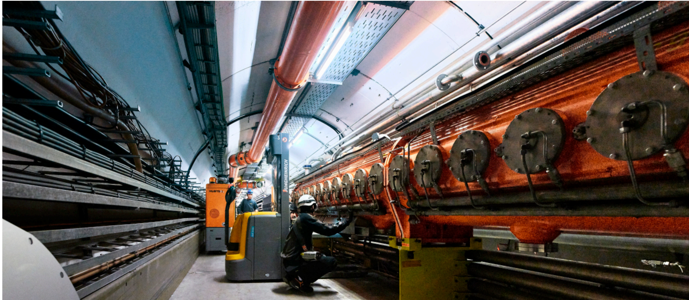
CERN-PHOTO-201902-032, SPS RF accelerating cavities removed from the tunnel of the accelerator
