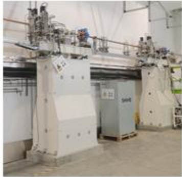
m-Magnet Support Platform
