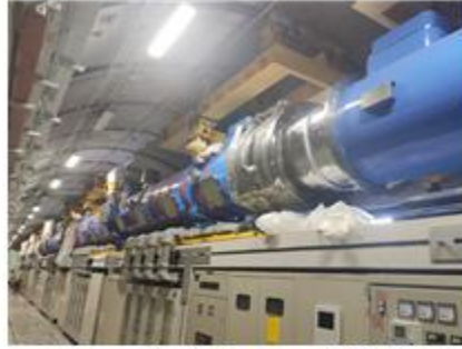
Suspended Support Platform of Cryomodule
