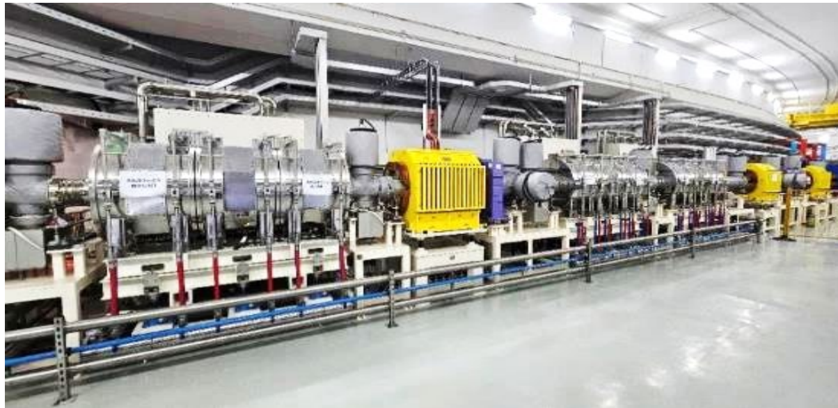
MA loaded RF system in the tunnel
