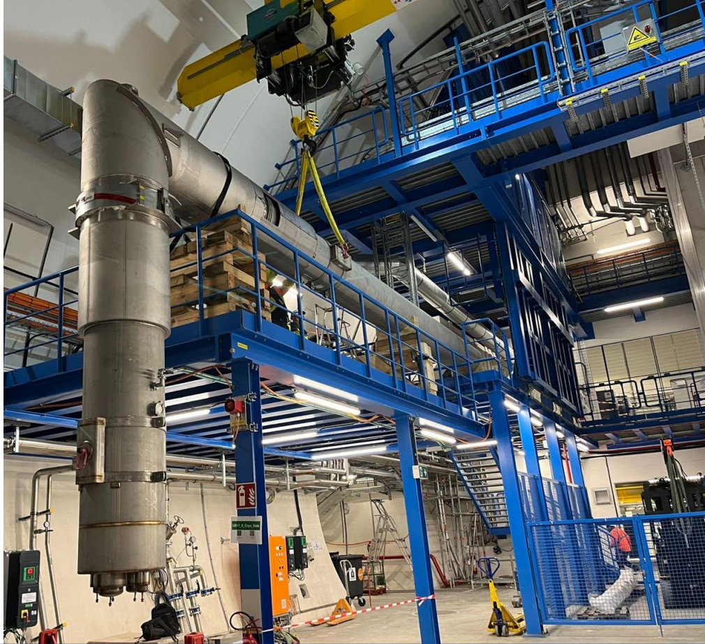
Lowering and temporary storage of first spools for connection to QPLG in Pt5
