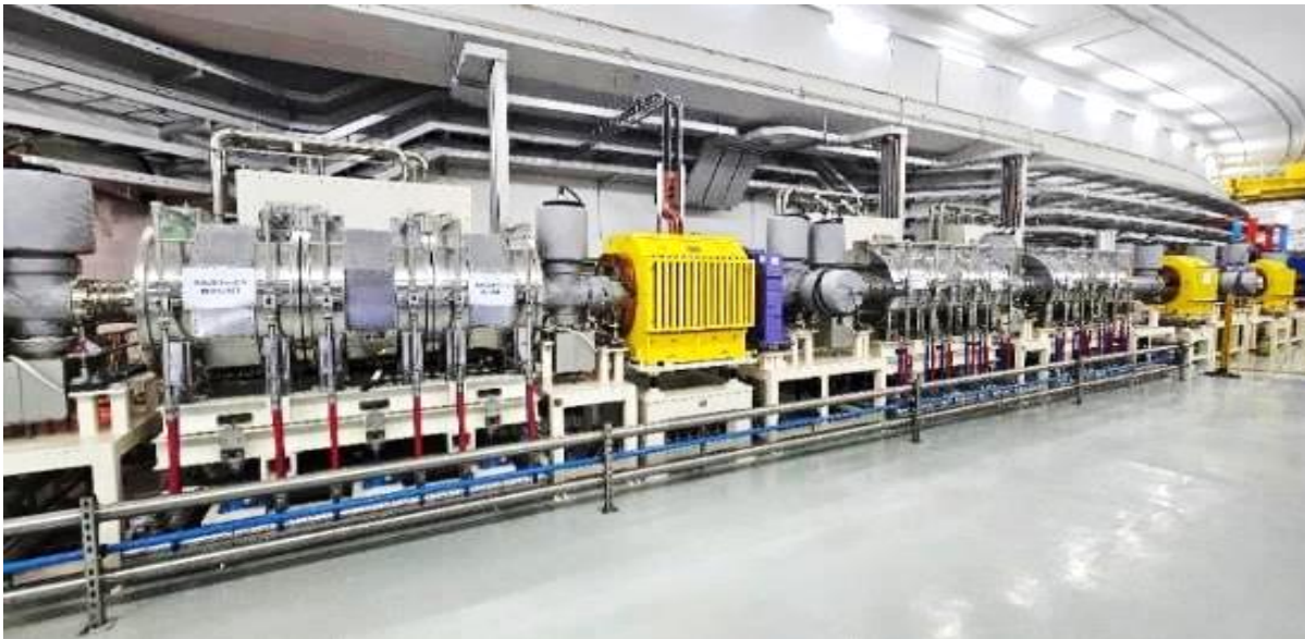
MA loaded RF system in the HIAF tunnel
