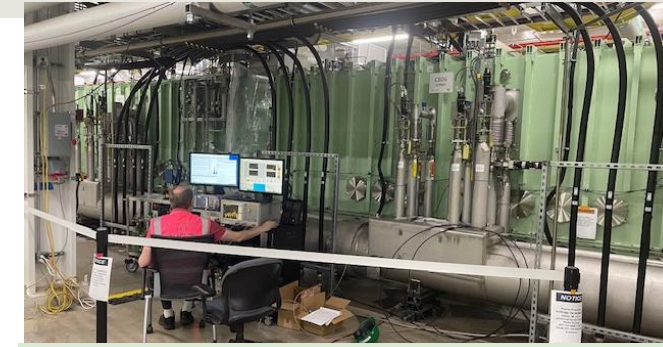
Plasma processing in the linac tunnel
