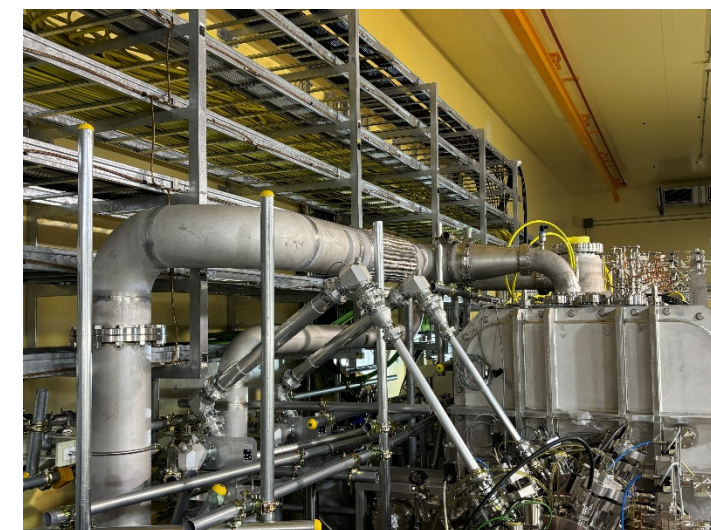
Safety outflow pipes
