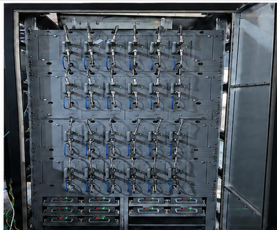
(a) 650 MHz / 70 kW SSPA System (Front View)
