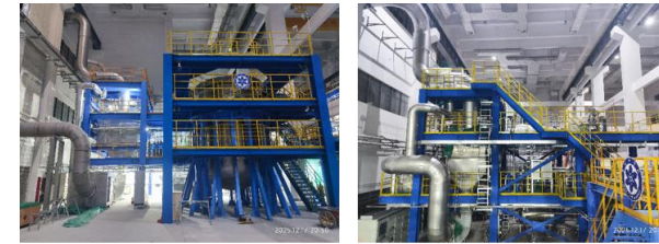
System View (Partial)
