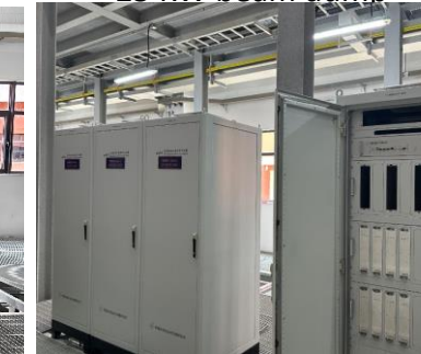
Power Supply System
